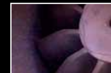
Exhaust fan blades using 6mm long focus camera (VSA2-1)
