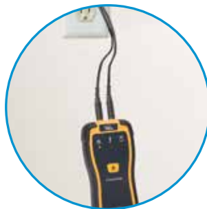
Traces on de-energized circuits
